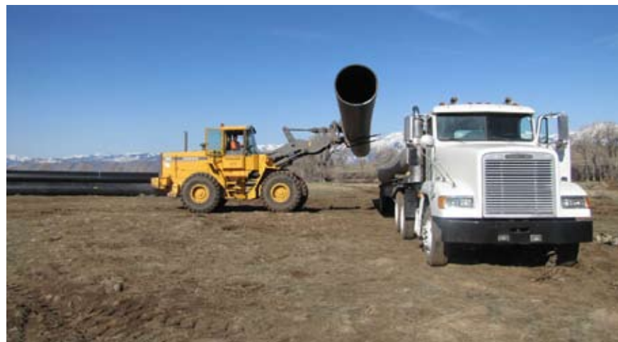
Large diameter pipe that was delivered to the Refuge in December is unloaded and piled at a designated staging area.
